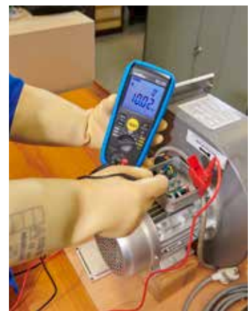
Preventive maintenance preventive on a motor
